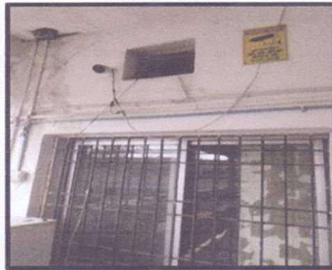
CCTV cameras in the college premises
