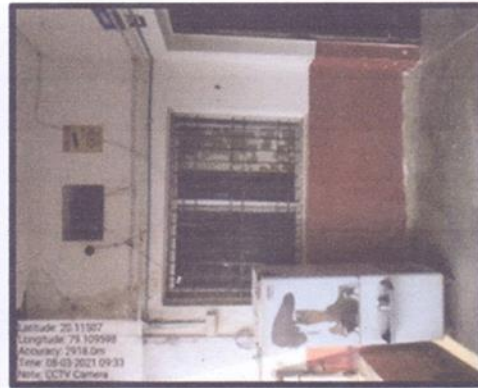
CCTV cameras in the college premises
